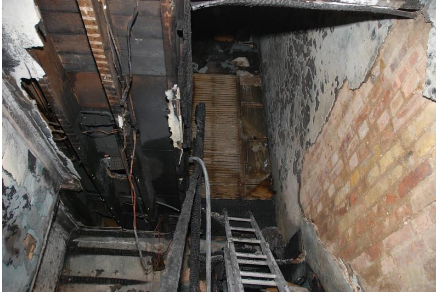
Following a fire under the stairs, the stair treads have burnt through, the ceiling has failed and the plaster has come off the wall.
