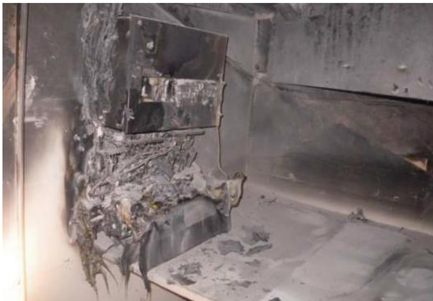
This photo shows a fire involving a plastic consumer unit (bottom) and a metal consumer unit (top). In the experience of the LFB, when a fire originates within a metal consumer unit (even without sealed grommet holes and the plastic MCB cover failing), the fire is still generally contained to the consumer unit.
